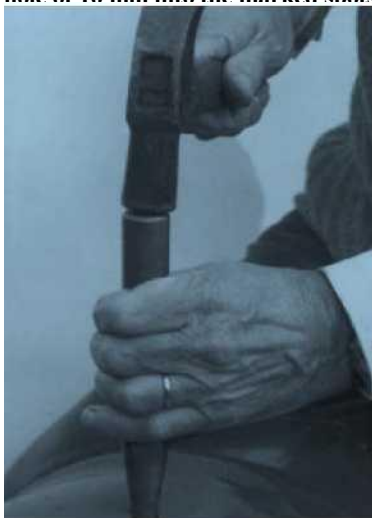
By using the steel cone and hammer widen one hole until a W piece of pipe fits in perpendicular of the drum
