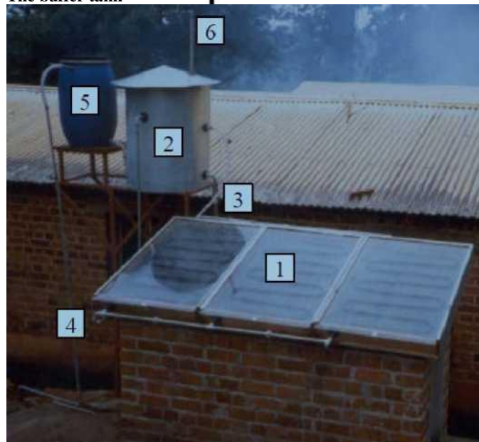
Complete solar water system
